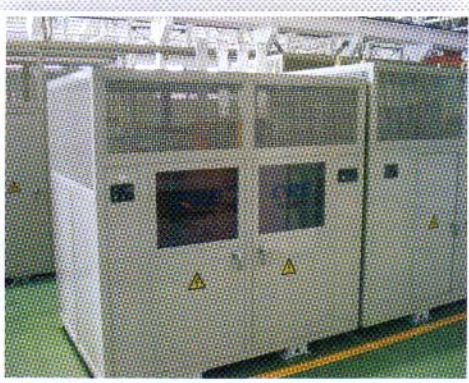
Transformer With Enclosure
