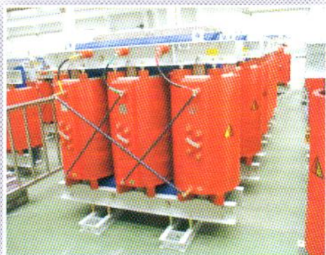
A View of 11 KV Cast Resin Transformers
