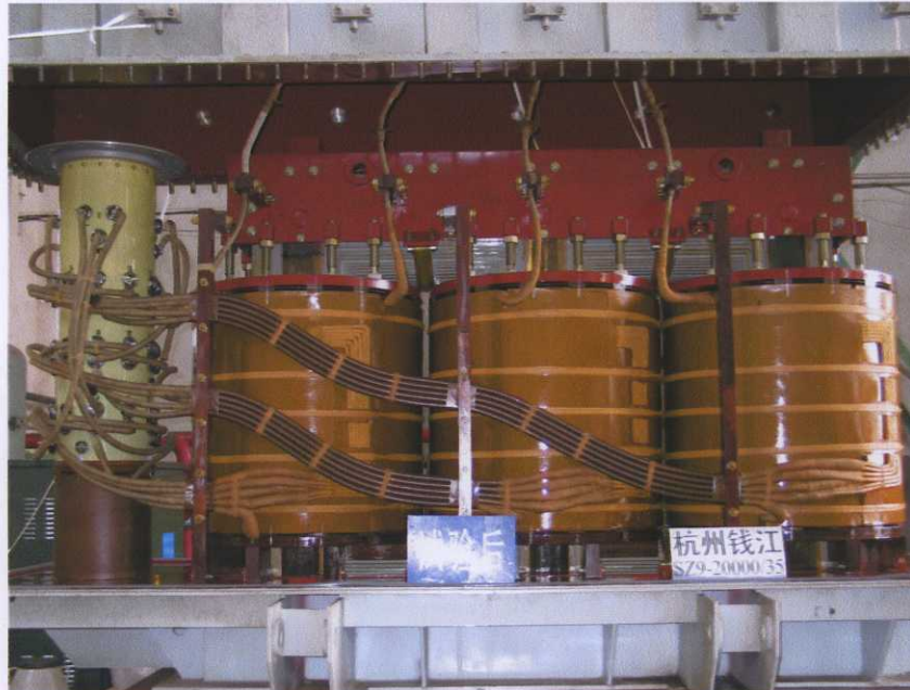
High voltage side after S.C.T.:
