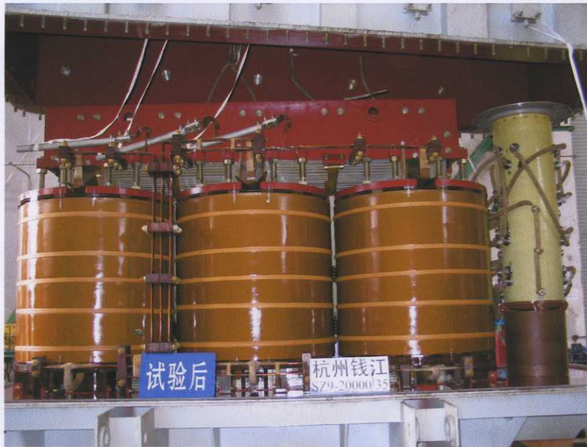
Low voltage side after S.C.T.:
